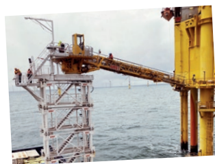
GANGWAYS (TELESCOPIC ACCESS BRIDGES)
